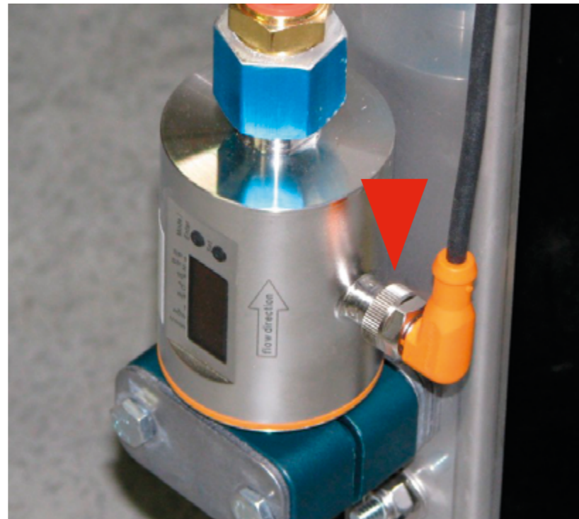
Signal cable connected to Flow Meter
