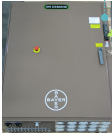
Main Control Panel
