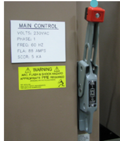
Main Control Panel Switch in ON position
