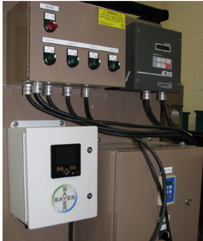
Flow Meter installed on old style 3-piece RH 4-pump control, ref.
